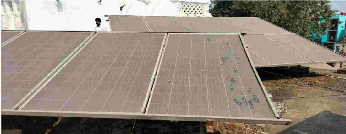
Fig: Grid connected Solar PV Plant at Office building
